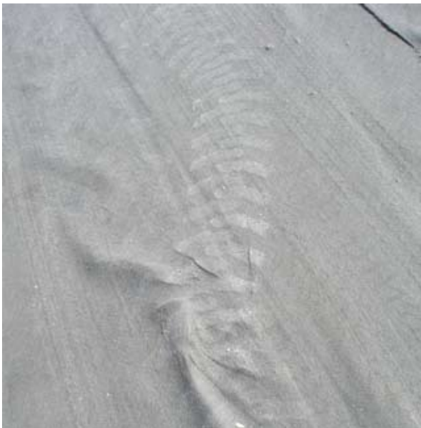
Figure 19. Localized shoving of geotextile due to short-radius truck turning maneuver.
